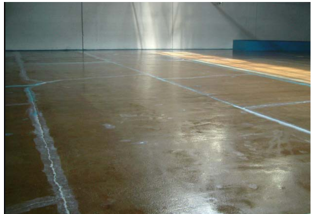
Completed surface preparation consisting of shot blasting, Retro-Coat Caulk, to fill joints and cracks and a 6 mil application of Retro-Coat Primer
